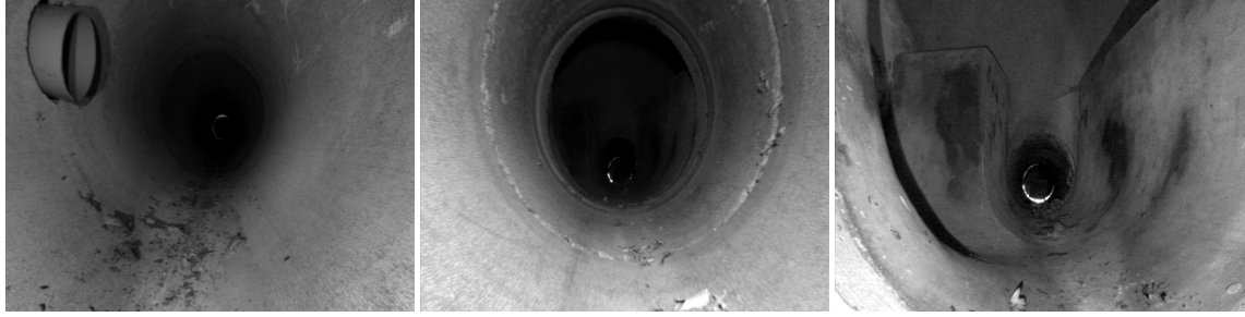
Fig. 2. Images of an inlet, pipe joints, and a manhole taken with MAKRO's cameras.
