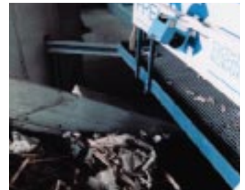
Bulk material measurement Refuse incineration
