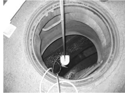
Figure 5b: View from aboveground into the underground utility caverns. ZLS07 is in the right vertical position and ready to acquire the environment.
