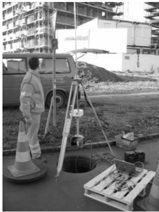
Figure 5a: ZLS07 is mounted headfirst to a telescope tripod system which guides the laser scanner into the underground utility caverns through a manhole.
